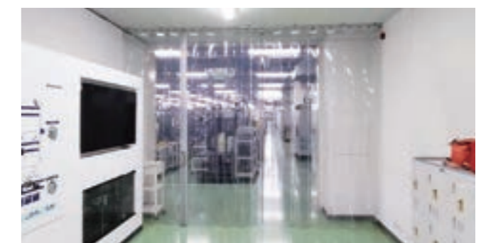
Vinyl curtains installed to reduce amount of electricity consumed by air conditioning
